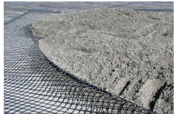
Geogrid 'buldge' In Advance of Fill Placement
